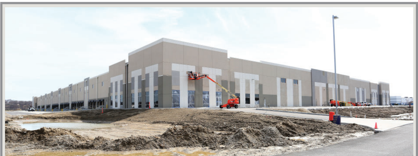
NorthPoint is under construction on HTP5, a 415,000 square foot speculative building and HTP1, a 250,000 square foot speculative building in Hazelwood.
